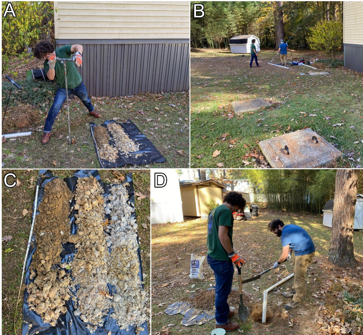
Figure 2. A) Will Shingleton (BS Environmental Health Student) augering a borehole. B) Access risers to the septic tank shown in the foreground while a piezometer is installed in the background. C) Soil profile laid out for soil analysis. D) Grouting the piezometer within the borehole.
